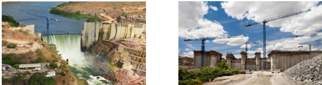
Image 3: COMANSA Cranes in the construction of the Baixo Sabor dam in Portugal (LEFT) and Cambambe power station in Angola (RIGHT)
